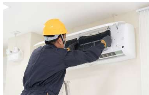
Air - Conditioning & Refrigeration
